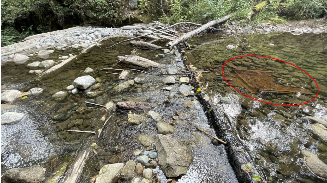
Photo 2 Low-Level metal intake grate and remnants of wooden flashboards, looking east (from left side of dam).
