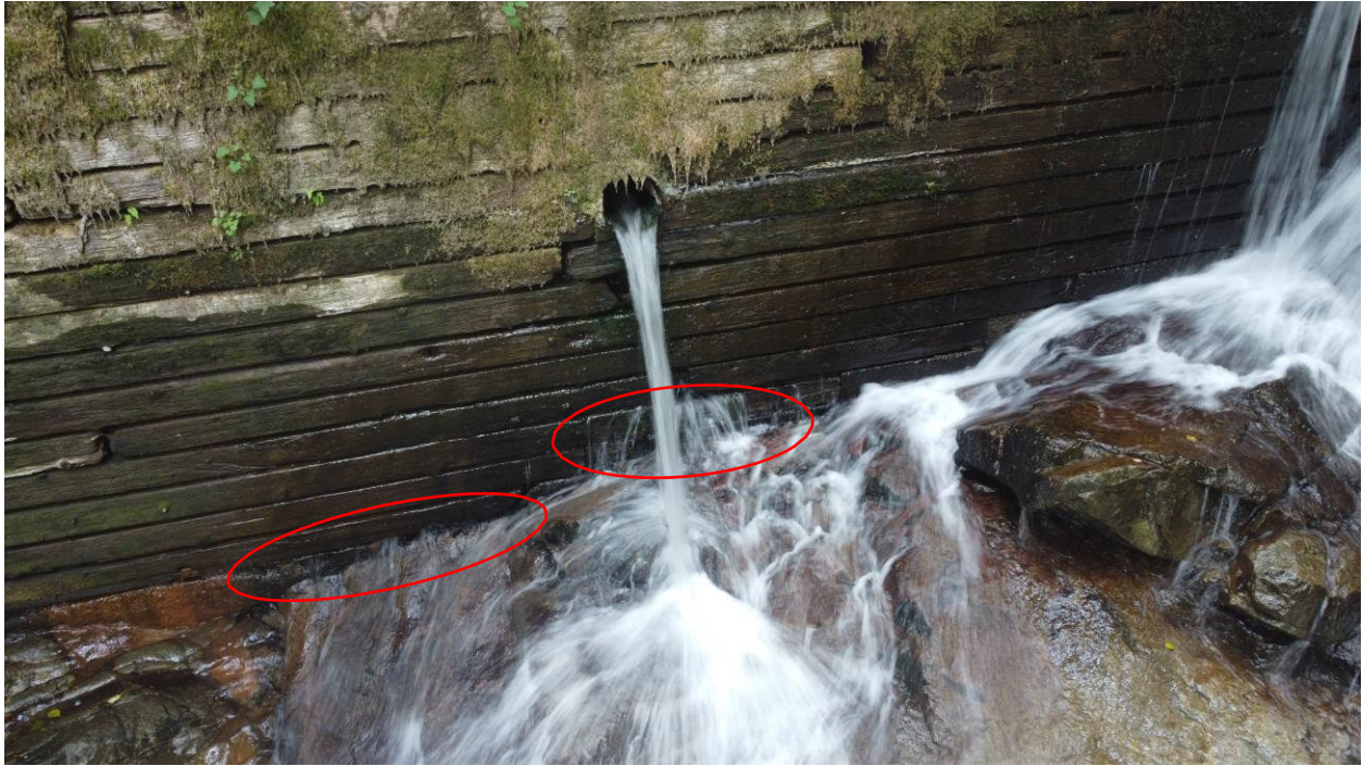
Photo 7 Major seepage at toe of downstream face.
