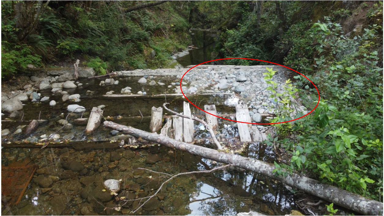
Photo 3 Top of dam with debris buildup on right side, looking northeast (downstream).
