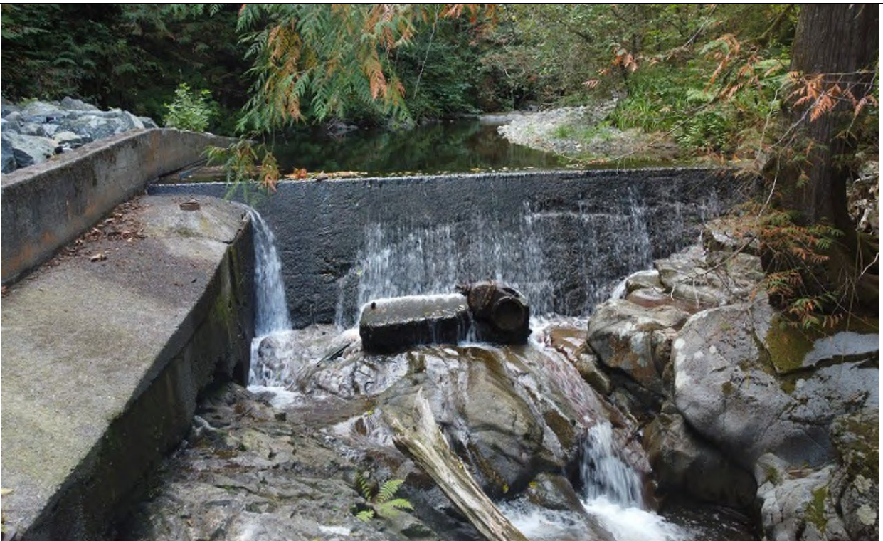
Photo No. 12 Date: 19 September 2023 Looking Towards: West Location: Water Supply Dam Description: Looking at Water Supply Dam during the low flow period.
