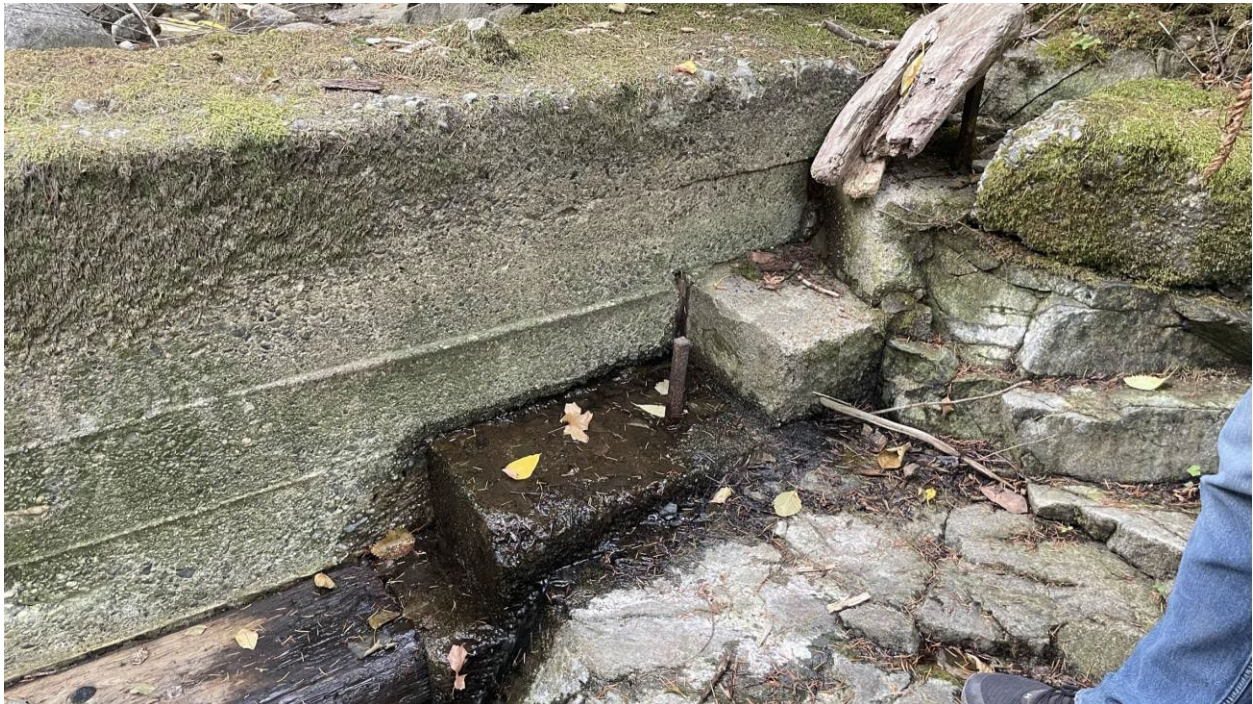
Photo 6 Seepage underneath left concrete abutment.
