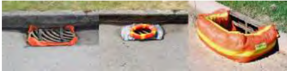
Figure 3. Catch basin inlet protection examples. From left to right: catch basin insert, donut and sediment log.
