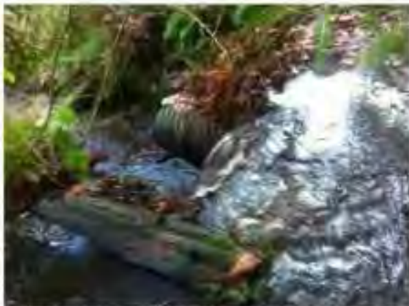
2.) Washed out culvert at old Hydro Rd
