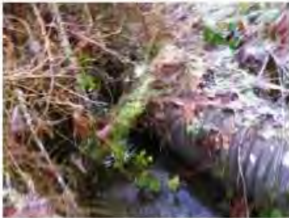
3.) Washed out culvert at old Hydro Rd.
